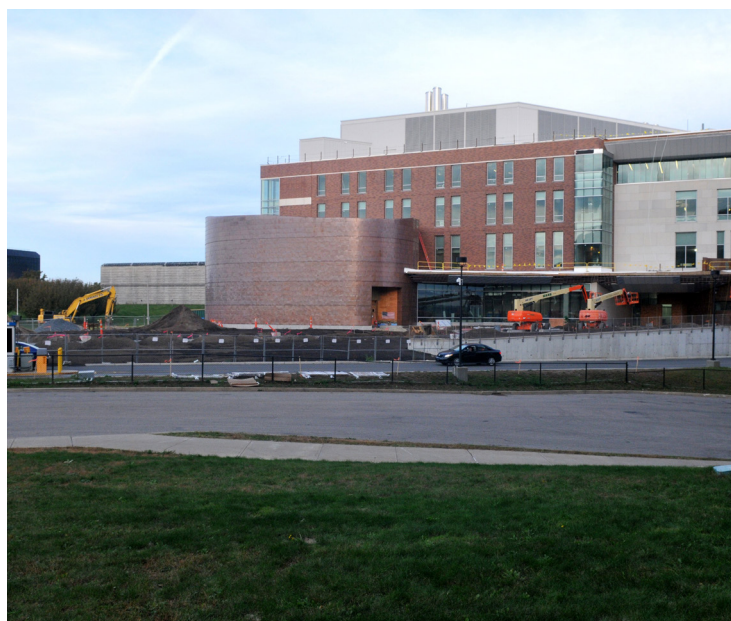
Crews continue making progress on chemistry, performing arts, and general classroom space at University Hall, which is scheduled to open in the spring.
